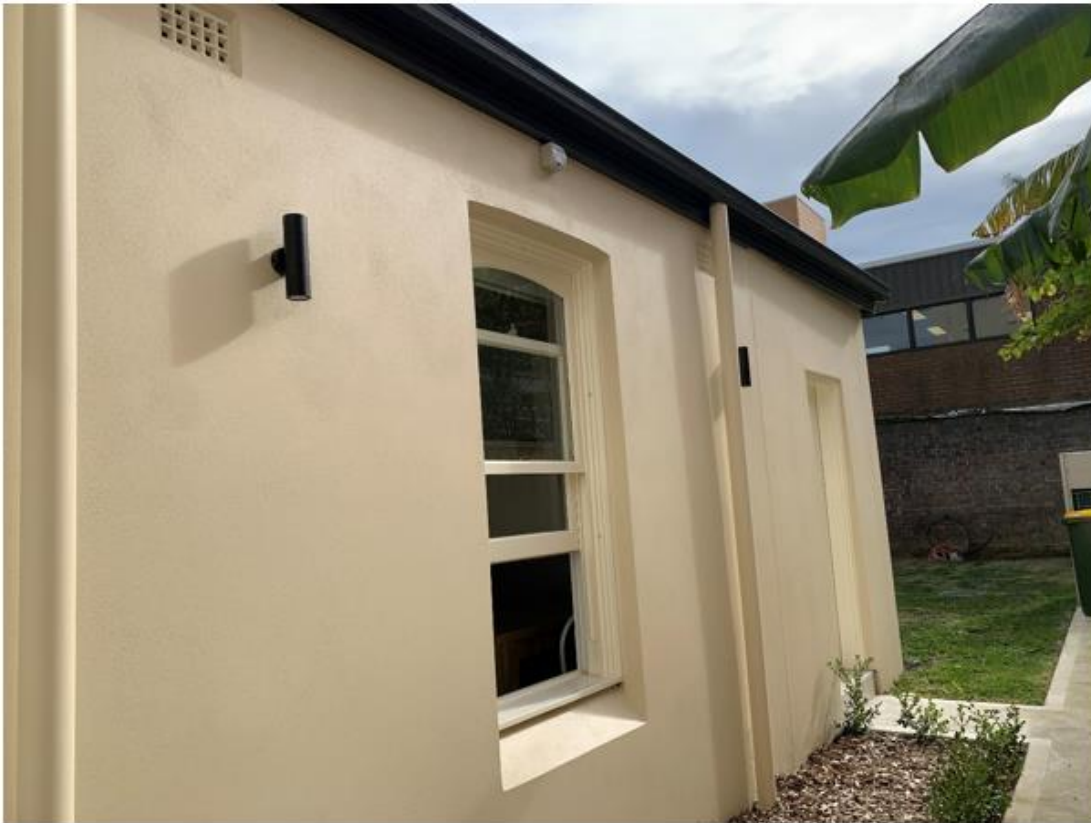
Figure 6: View towards the north eastern facade of existing rear wing and to the rear yard beyond
